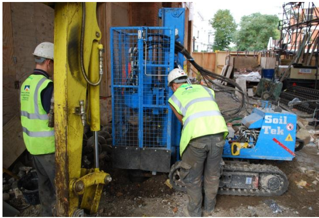
Fig 19: All mini piling rigs must be guarded around the auger head to comply with HSE requirements
