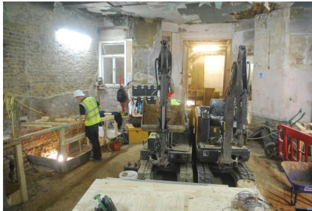
Fig 20: Larger projects can use mini excavators to assist with carting “muck away” and excavating
